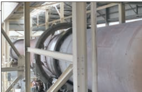
FIGURE 3. A view of a refractory lined kiln for producing proppants is shown in this photo
